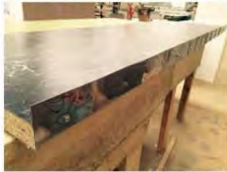
Stainless steel plate fixed in position to bench top
