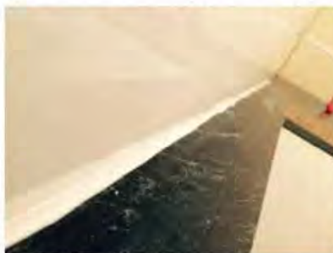
New splashback is to be laminated on all edges to stop water penetrating splashback. Excess sealant is removed on completion.
