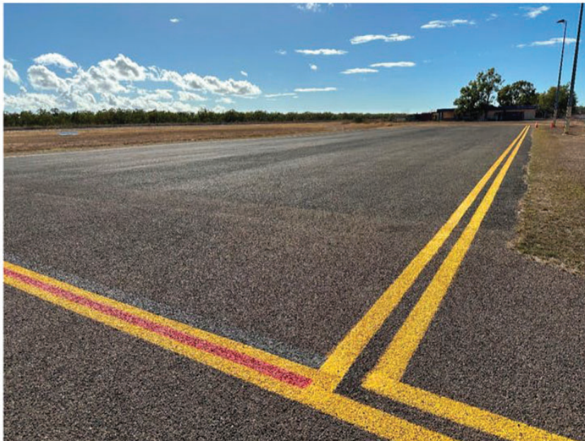
Photograph 7. Similar condition of the GA Apron.
