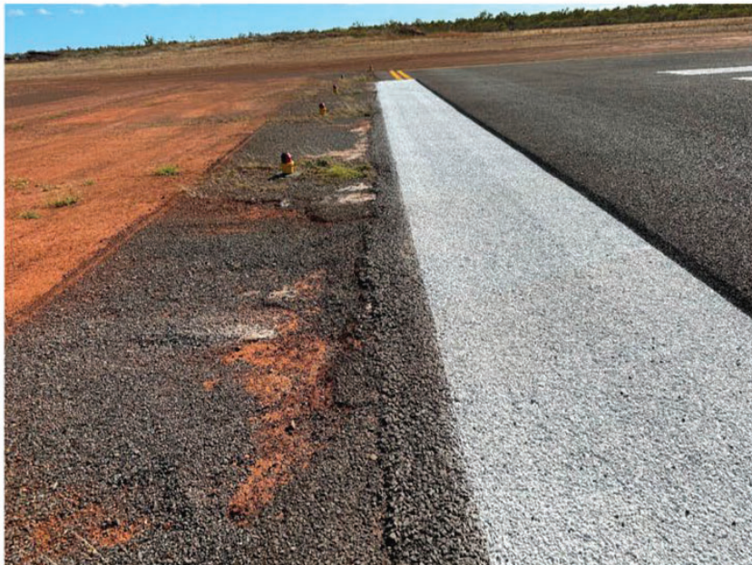
Photograph 3. Example of edge break aways at the runway end.
