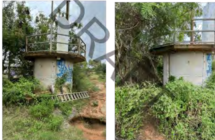
Figure 14: SPS C Compound
