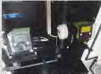
New duty standby chlorine dosing pumps
