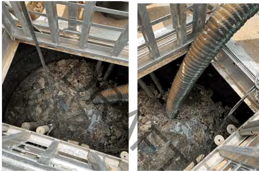
Figure 6: SPS A Wet Well
