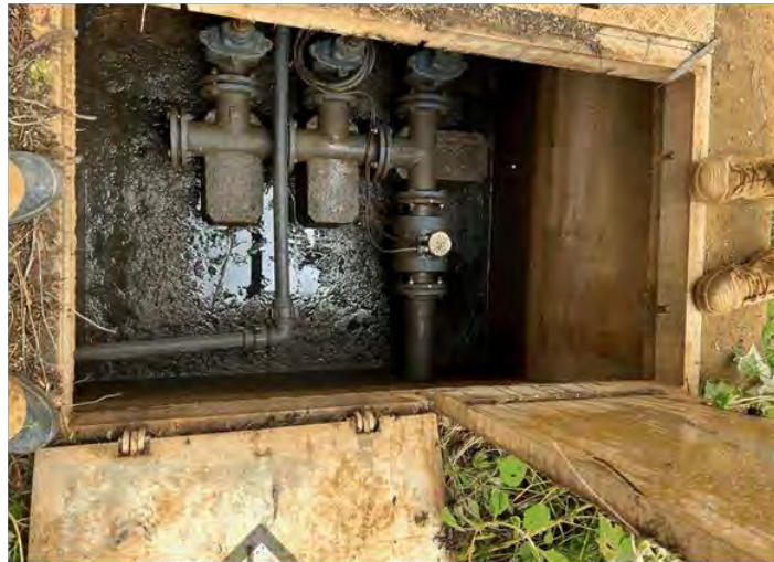
Figure 16: SPS C Valve Pit
