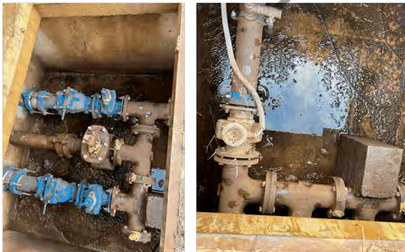
Figure 12: SPS B Valve Pit
