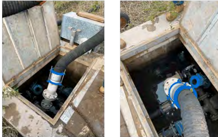
Figure 7: SPS A Valve Pit
