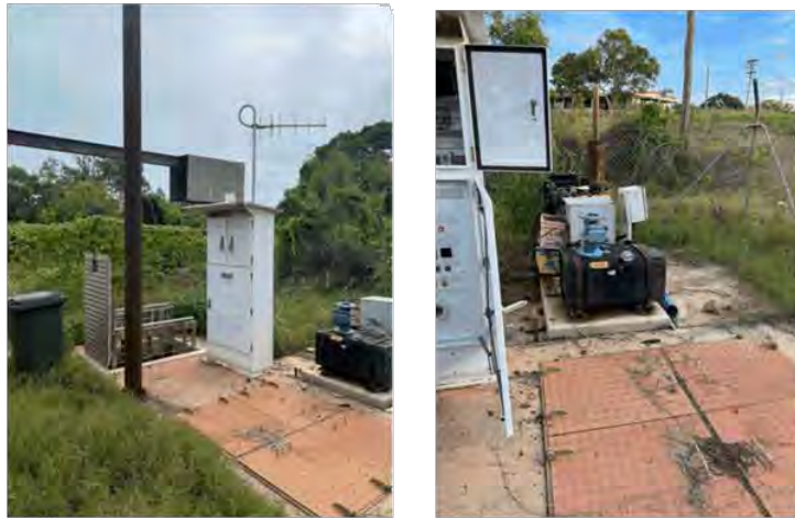
Figure 10: SPS B Infrastructure
