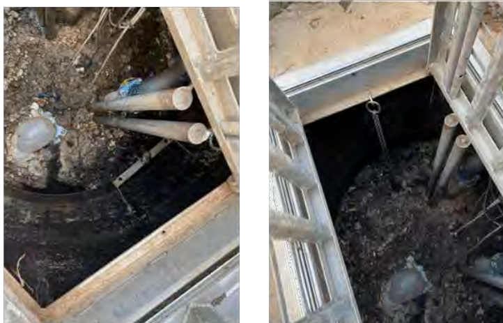
Figure 11: SPS B Wet Well
