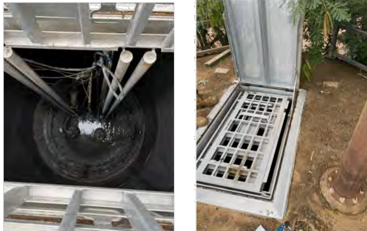
Figure 15: SPS B Wet Well
