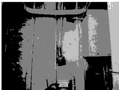
CORROSION UNDER BRIDGE
